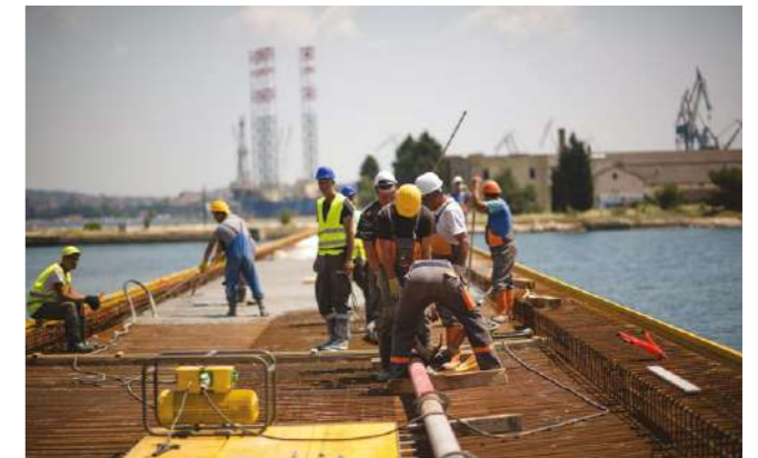
Armiranje nove proširene ploče mosta Bridge deck reinforcement for a newly expanded bridge
